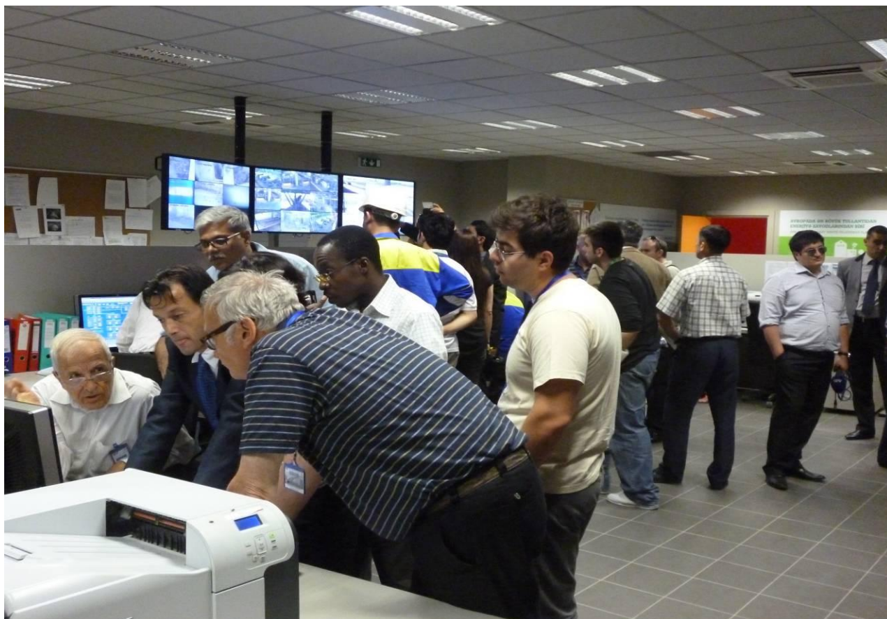
Phot. 14. Control Room WTE Plant Bakou
